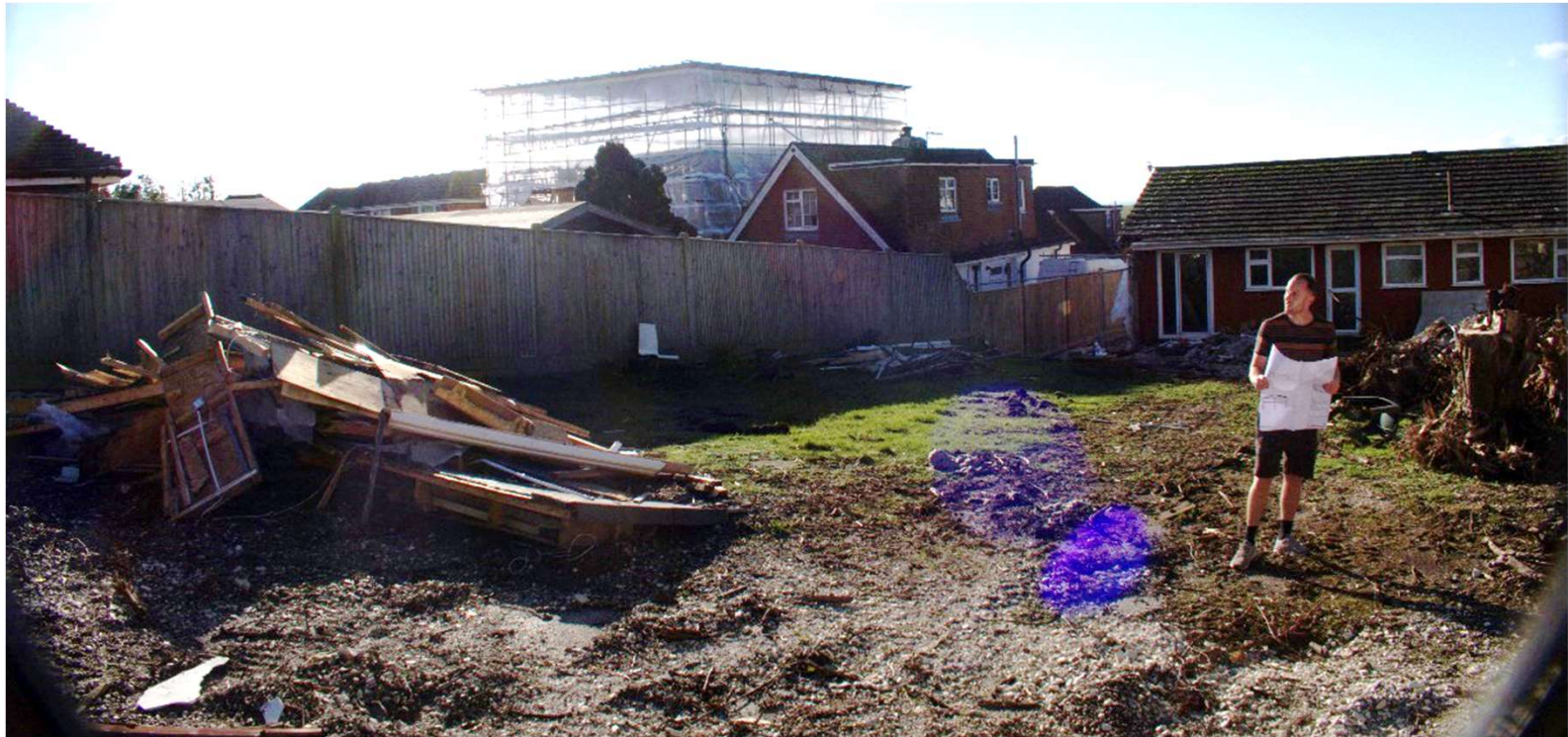
View from the northern rear corner of the site, looking towards rear of pre-existing bungalow and southern side boundary
